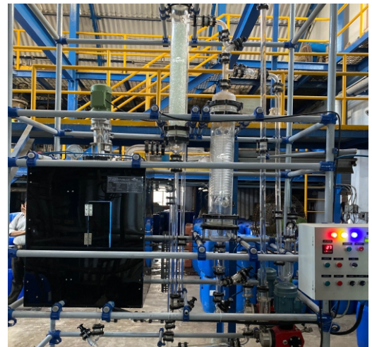
Continuous Photo-Chlorination Unit
